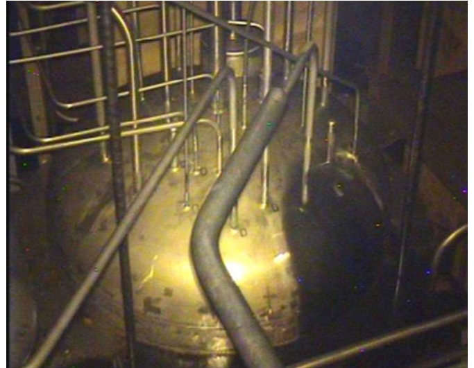
Figure 6: Top view of a vessel in cell, showing pipes entering the vessel
